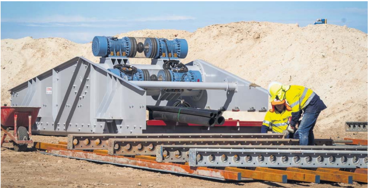
The first screen being delivered to the Bald Hill site, near Kambalda. Picture: Tawana Resources
