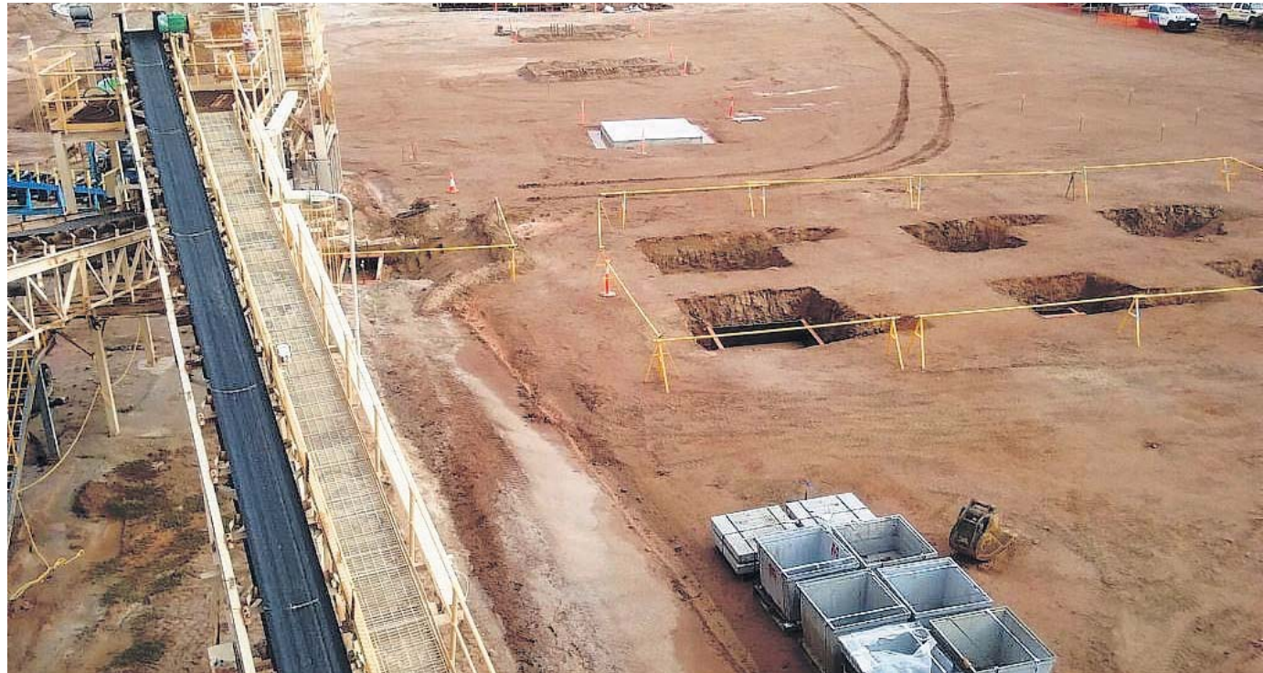
Construction is under way at Tawana Resources and AMAL's Bald Hill Lithium Mine south-east of Kambalda. Picture: Tawana Resources
